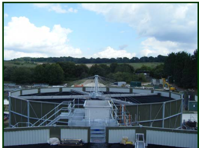
HYCOVER Distributors safely installed.
