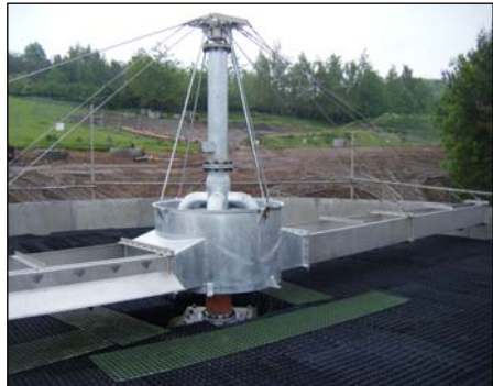
Twin trough arm HYCOVER rotary distributor with variable speed drive arranged to apply up to 70lt/sec of primary settled sewage to the surface of a 13.1mt Ø roughing filter containing some 430m 3 plastic media packed to 3.6mts
