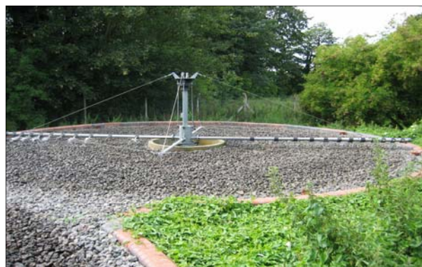
2 Arm reaction driven HYCOVER 'Lo-Flo' tubular arm distributor applying 3.2 lt/sec to an 18.0 mt dia stone trickling filter.
