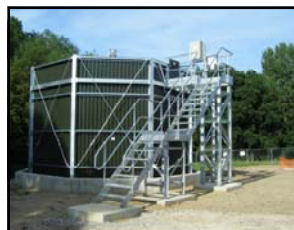
Typical HYRATE Polytower with stairway and local control panel on top platform adjacent to doorway.
