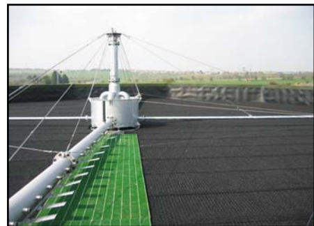
Twin tubular arm HYCOVER rotary distributor with variable speed drive arranged to apply up to 60lt/sec of secondary sewage effluent to the surface of a 22.5mt Ø HYRATE Polytower packed to 6.0mts with some 2430m 3 of modular plastic media
