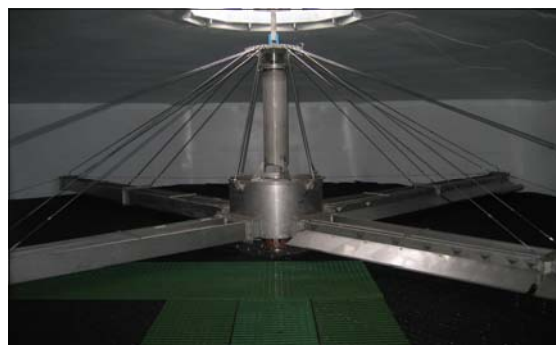
4 Arm all stainless HYCOVER trough type machine, to apply 55 lt/sec of primary sewage. Fitted with external over-mounted variable speed drive. Installed in an 11.75 mt HYRATE Polytower fitted with roof and low level odour extract system.
