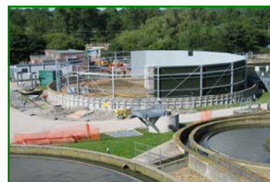
New 25 mt dia Polytower filter shell under construction using timber matrix as a working platform and for storage of materials.
